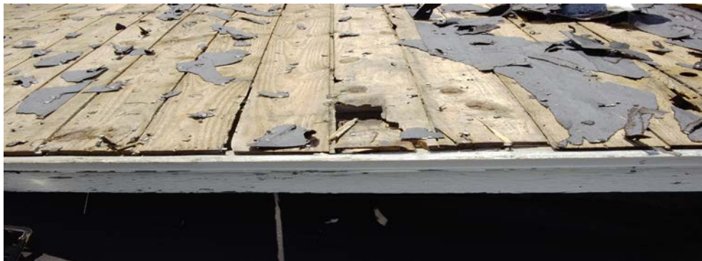
Older Deteriorated and Damaged Deck (Board Decking)
